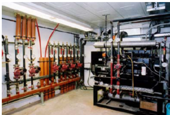
Figure 5: Example of a combined heat and power plant [Source: Biogas-Nord/ENSPAR Biogas]
